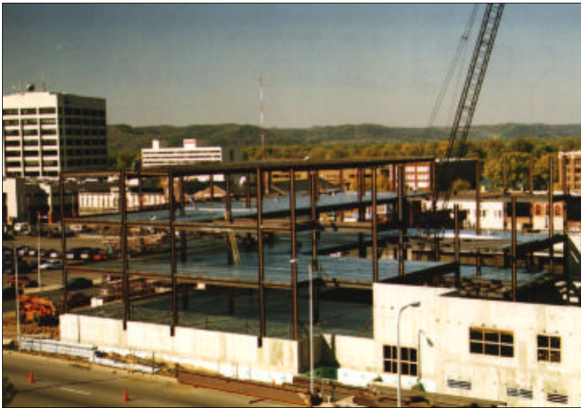
Construction began on a new courthouse in La Crosse County in 1996. The building meets the standards on security and facilities set forth in the Supreme Court Rule. It houses the courts, district attorney and clerk of circuit court, and will adjoin a new jail. The building was completed in August 1997.
